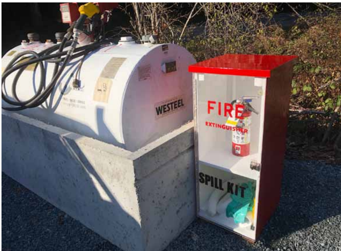
Cement-bermed diesel tank and spill kit
