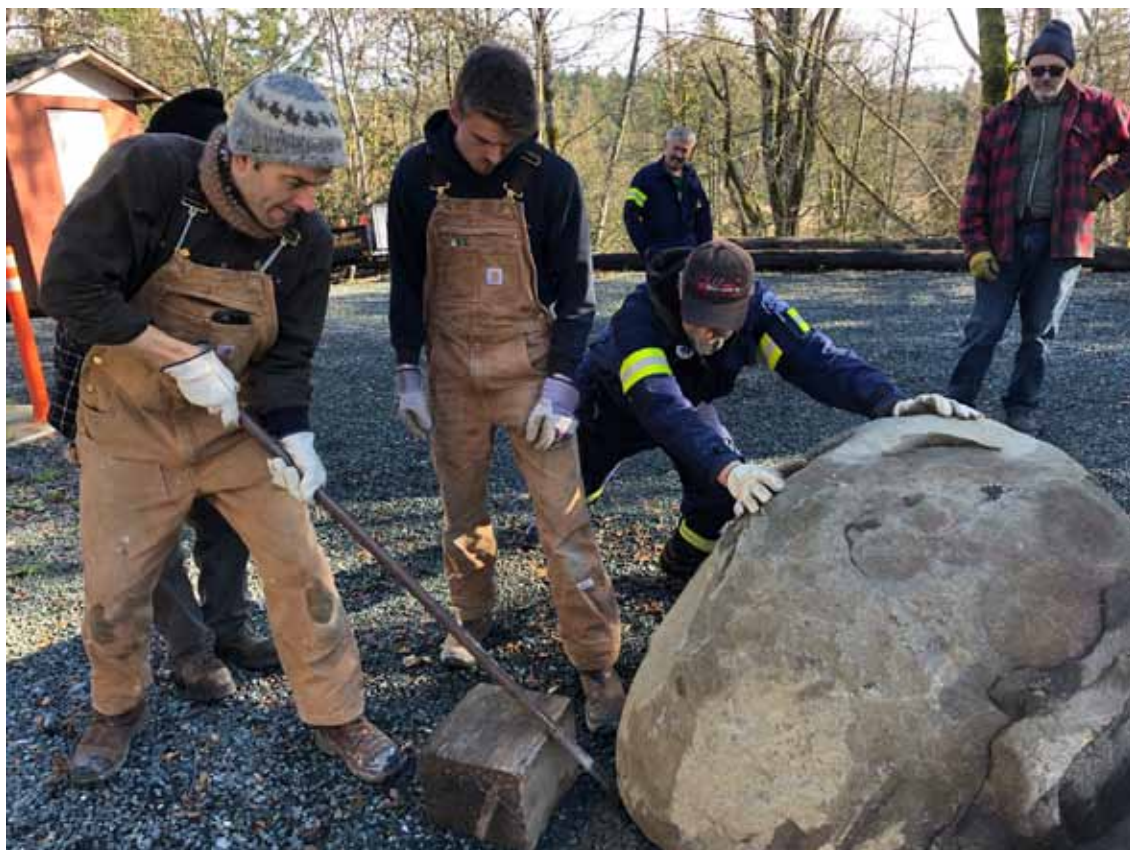
February 2020 - among the last of the maskless work parties, clearing the way for the concrete apron around the new Fire Hall.
